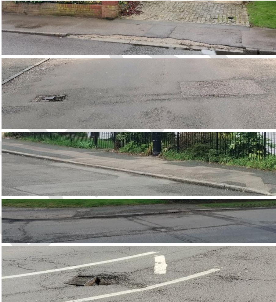
Fig. 5.4: Examples of poor road and pavement surfaces
